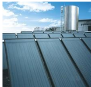
a) Flat plate collectors
